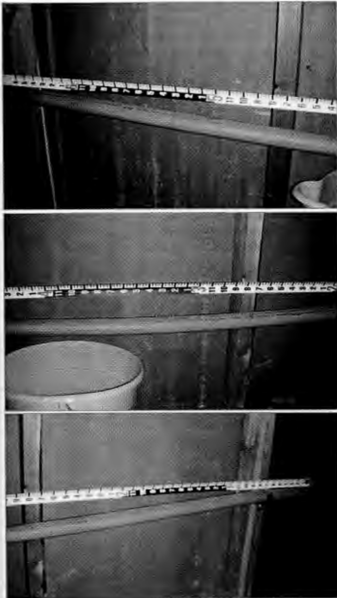
Figure 6 – Sagging of an installed CPVC pipe exposed to a mixture of water and bio-glycerin.
